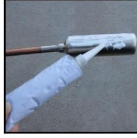
11. Smear silicon grease on the surface of het pipe condensor. (Used to increase energy transfer efficiency)
